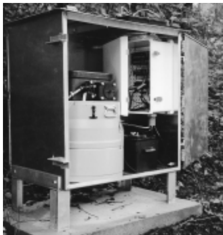
Riverkeeper's first real-time monitoring station
